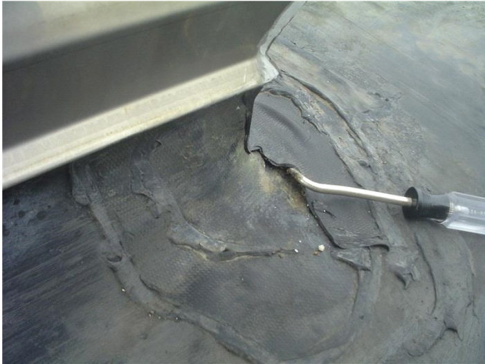
01 Hole in Flashing- Before
