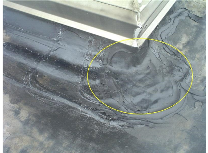
02 Hole in Flashing- After
